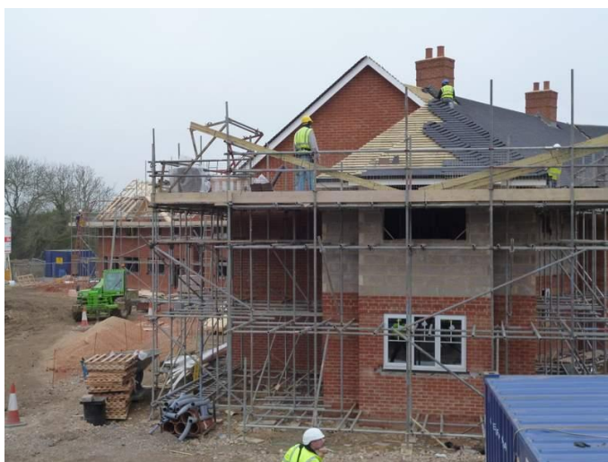
Photo 4: Work in progress on 32 affordable homes which will be owned and managed by Sentinel (March 2012)
